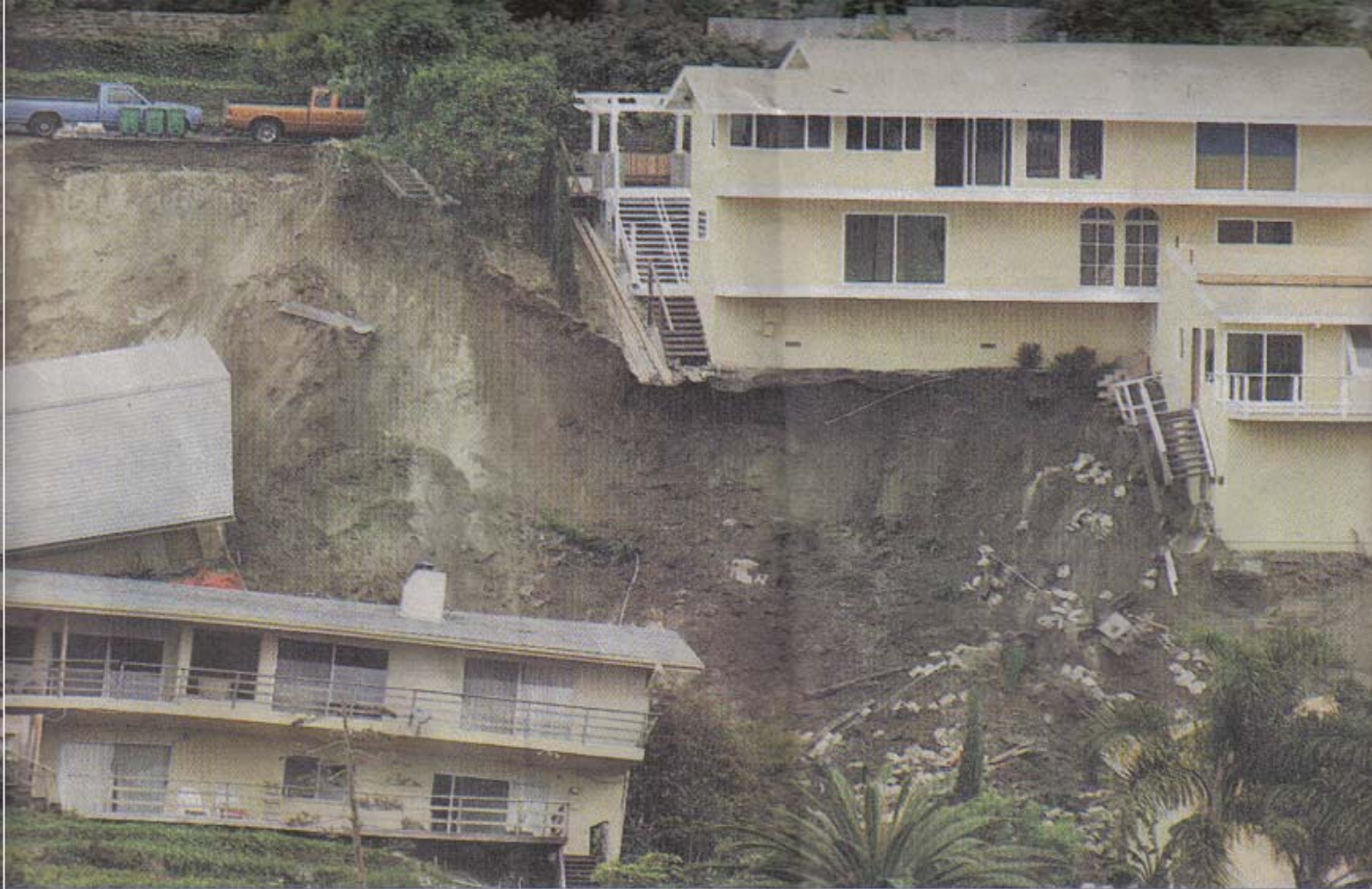
Houses sit knocked off their foundations after an early morning landslide in Laguna Beach, California. Police said 17 homes were destroyed or seriously damaged, and about 11 others were destabilized by the slide. Many of the homes slid intact down the hillside, while some luxury mansions actually cracked in half.
