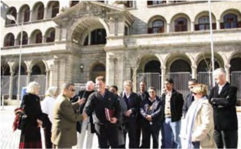
The R63-million DPW project to convert the former National Mutual Building into the Iziko Social History Resource Centre gets under way with the handing over of the building to the contractors.
