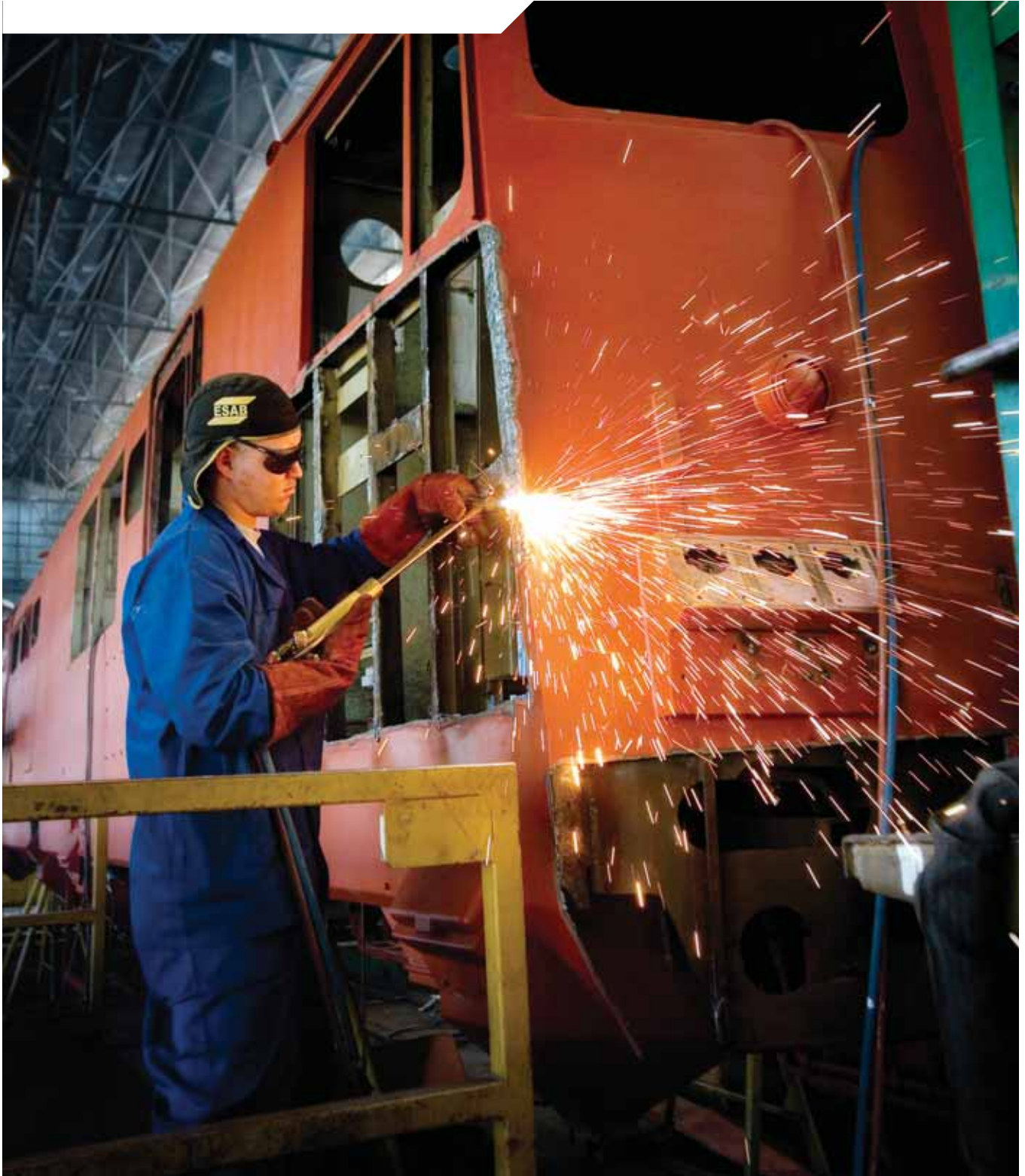
Rail Engineering's Vandyksdrift wagon maintenance depot received the highest safety award for the eighth consecutive year
