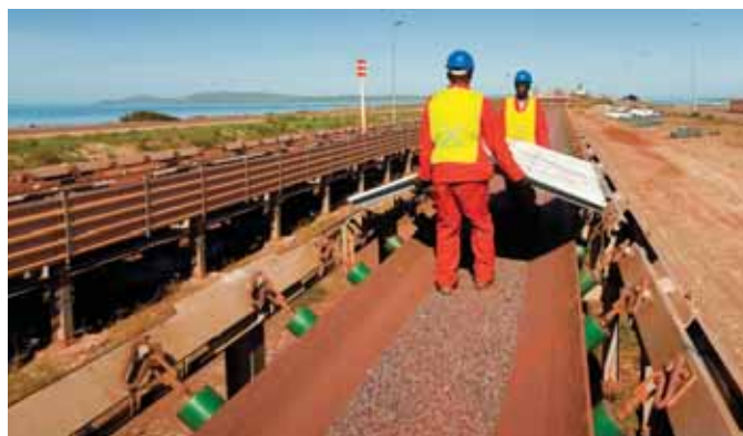
Dust covers are being put into place at Saldanha's iron ore terminal.
