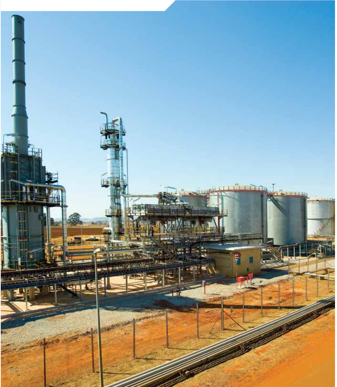
Transnet is investing nearly R10 billion to build the new multi-product pipeline between Durban and Johannesburg
