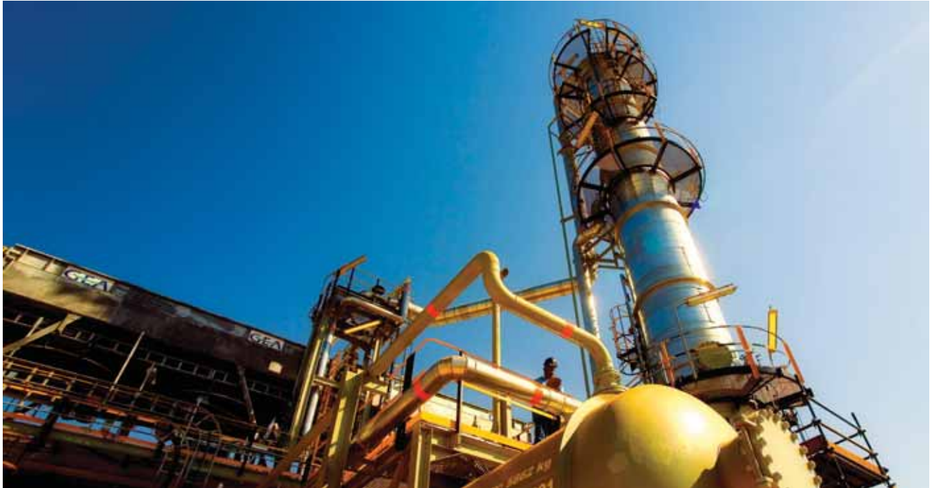
Pipelines' network of pressure pipes pumps close to 17 billion litres of petroleum products and 14 million gigajoules of gas per year
