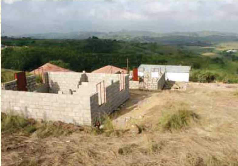
The Isimahla Rural Housing Project under construction during the year on Trust land at Vulamehlo
