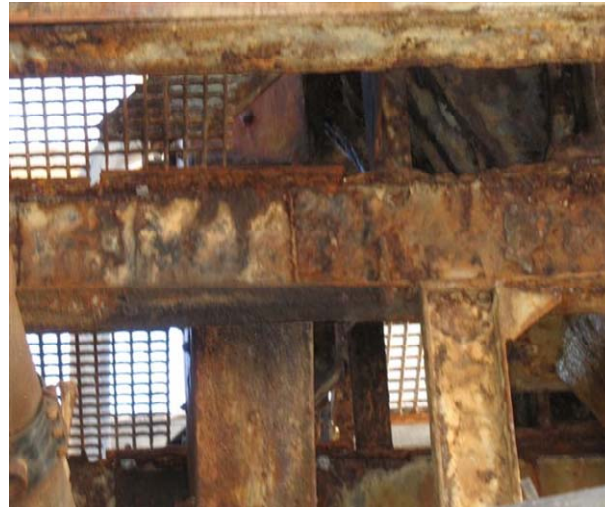
Corroded Steel Structures
